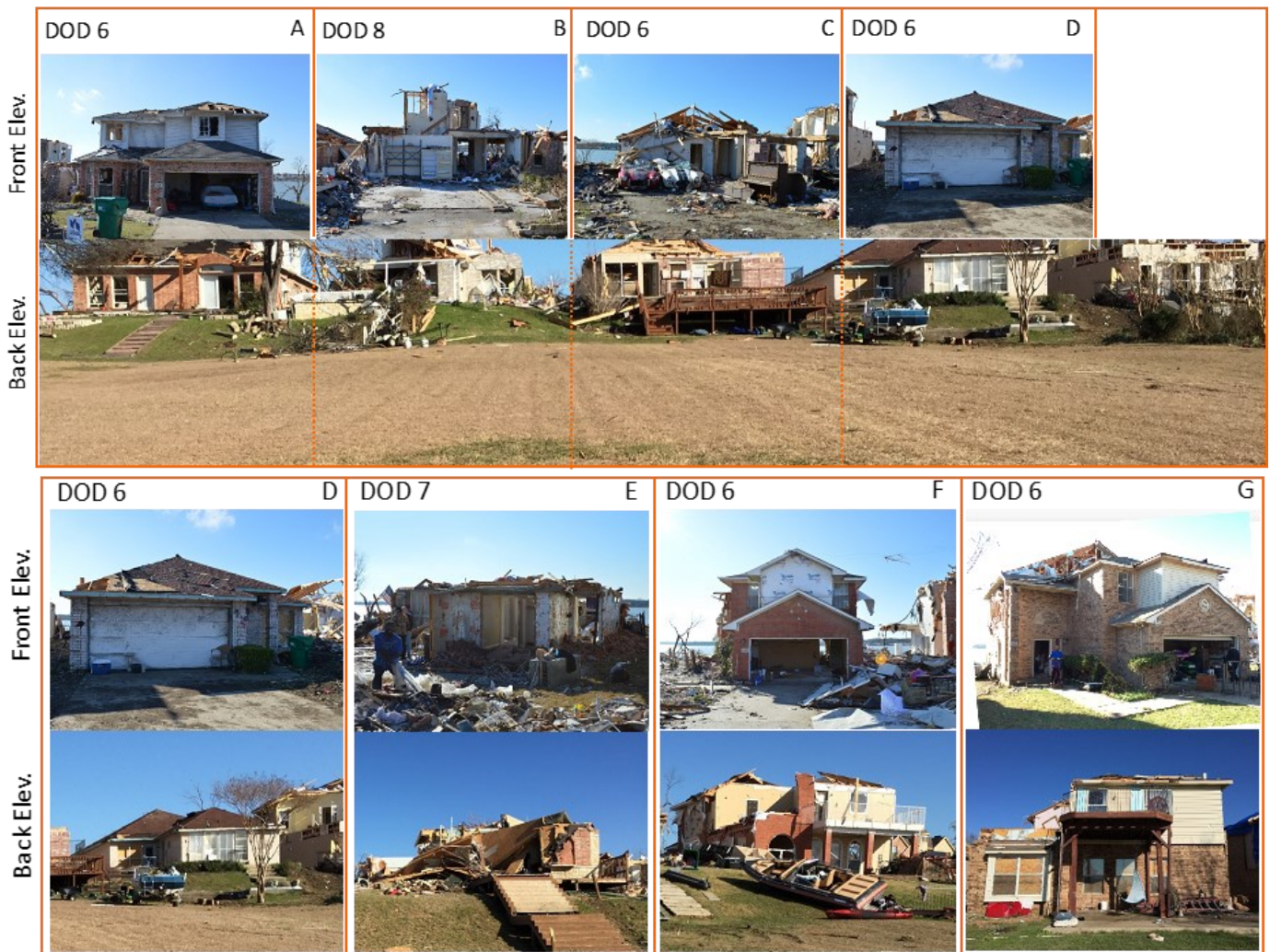
Figure 5. Typical damage and DoD Ratings for eight houses on Windjammer Way, Rowlett, TX. These waterfront houses likely experienced maximum wind speeds.
