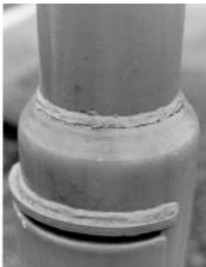
Figure 9. Fatigue failure in a lighting pole [33]
