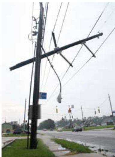
Snapped wooden poles add to local outages.
